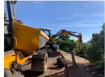
Damaged path and part of the road removed
